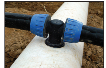
DRIPLINE SECURED TO THE TEE START CONNECTOR
